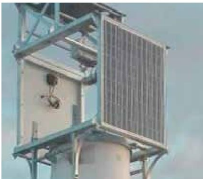
SOLAR PV SYSTEM
